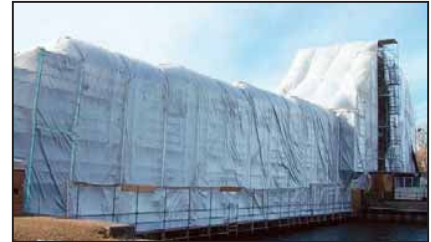
The LaSalle bridge carries 23,000 vehicles a day, as well as marine traffic passing below. Restoring and repainting the structure was a major logistical challenge.
